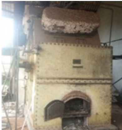
Figure 2: Outdated conventional kiln water boiler.
