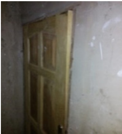
Figure 3: Warped panel door.
