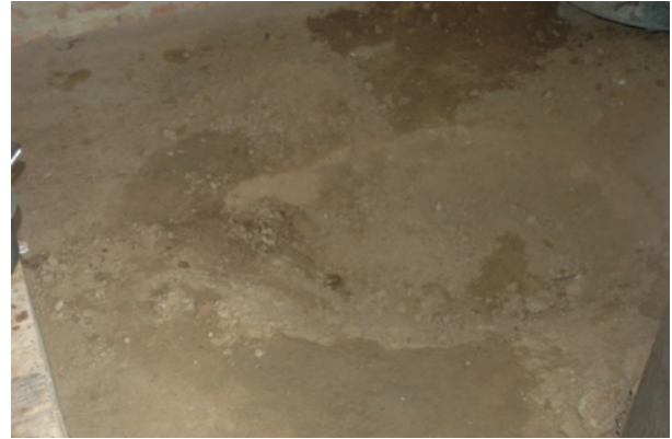
Figure 2: A fresh soil removed about 3 feet dip hole in the room floor.
