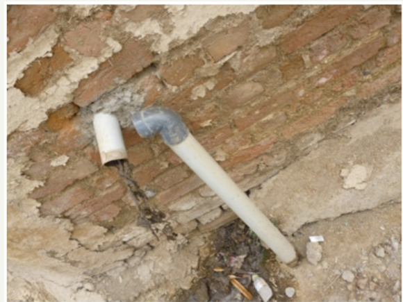
Figure 6: Outlet of P.V.C pipe from the deceased house.
