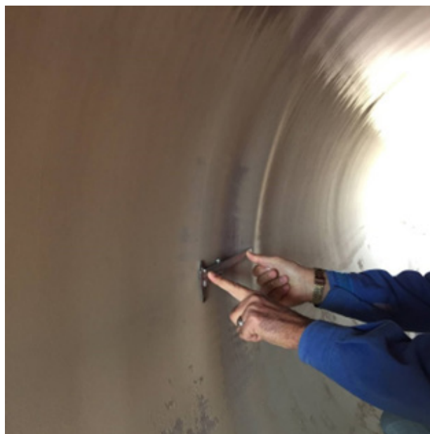
Figure 1: The inner side of the gas pipe.
