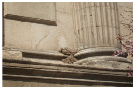
Figure 5: Pigeon feces accumulation at the base of a corinthian column, in the colonnade of the Iglesia de Santa María, in Alcalá de Henares (Spain).
