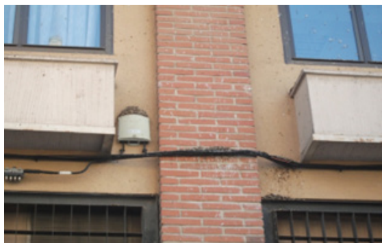
Figure 6: Swallow droppings accumulation over installation elements on the facade of a residential building in Toledo (Spain).
