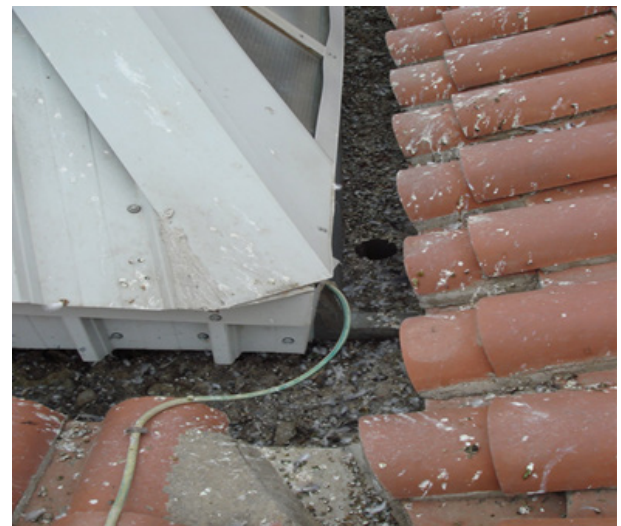
Figure 10: Detail of the roof of a residential building. The presence of birds can lead to the accumulation of a large amount of droppings and feathers, in addition to the birds that die on the roofs, which can clog drains and gutters, causing leaks and other damage.
