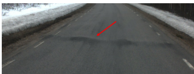
Figure 4: Positive culvert movement from road BD841. The picture is taken on road BD841 at section 46797 with an IRI measuring vehicle and is provided by Ramboll.
