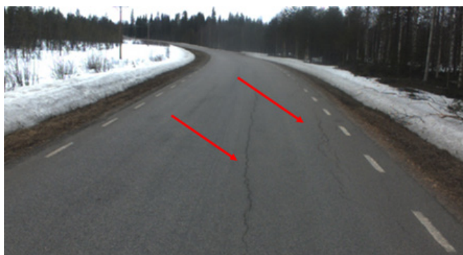
Figure 3: Cracks in wheel tracks caused by bearing capacity failure. A picture is taken on section 46607 on road BD841 with an IRI measuring vehicle and is provided by Ramboll.
