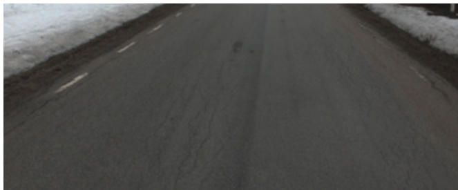
Figure 2: Micro-cracks in the pavement caused the bearing capacity failure. The picture is taken at section 46082 on road BD841 with an IRI measuring vehicle and is provided by Ramboll.
