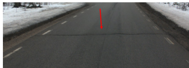
Figure 6: Temperature crack. The picture is taken on road BD841 at section 51409 with an IRI measuring vehicle and is provided by Ramboll.
