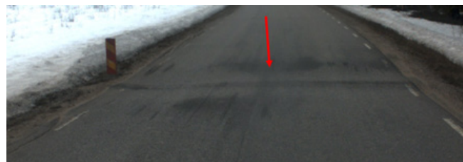
Figure 5: Negative culvert movement. The picture is taken on road BD841 at section 50499 with an IRI measuring vehicle and is provided by Ramboll.
