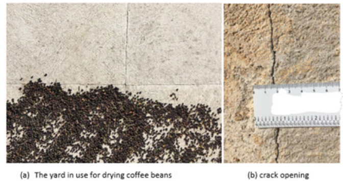
Figure 5: Cracks in the concrete patio.
