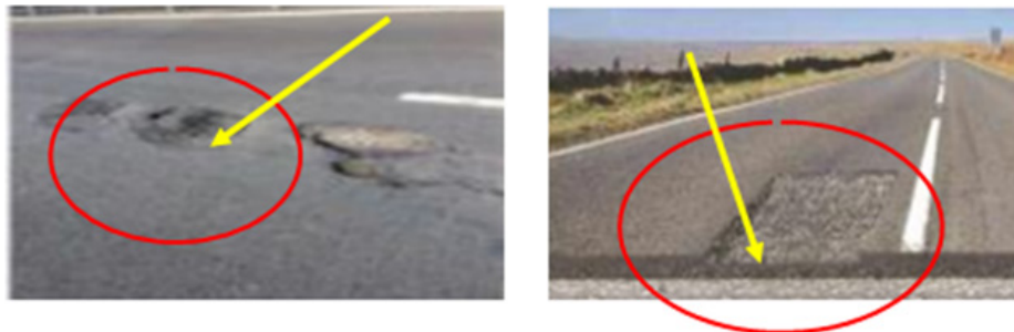
Figure 1: Damages to the wearing surface.
