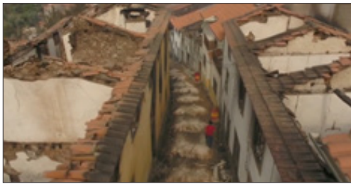
Figure 1: Example of old houses in which the roof burned, adapted from Portuguese press SIC.
