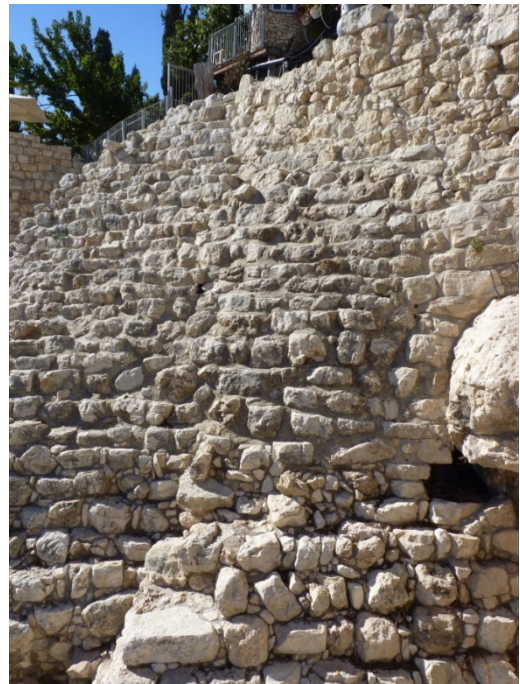
Figure 5: Part of the stepped-stone structure (Millo), which ranged upwards to stabilize the friable fill on which the early constructions of the city of David were situated.
