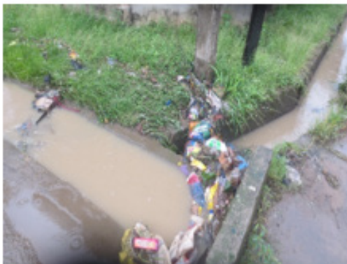
Plate 5: Poor drainage system in Urua Ekpa
